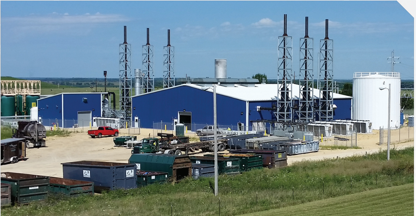
Orchard Hills Landfill Methane Gas Plant
